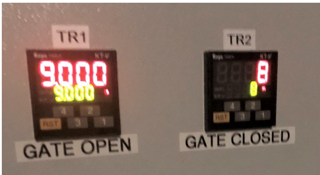
FIGURE 9: GATE TIMER OPEN AND CLOSED ON THE CABINET
